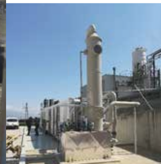
Scrubber system for emission abatement ↓
